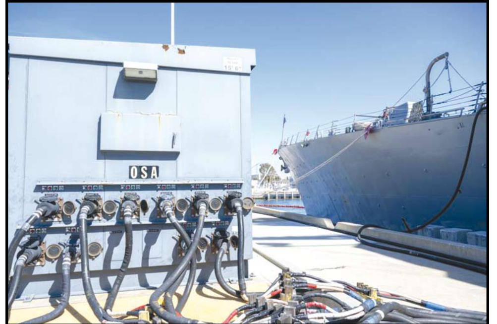
Ships moored at Naval Base San Diego are tied into shore power via cables and mounds on the pier. These power mounds allow the ship to power down its engines and run its systems on shore power. This reduces emissions from the fuel burning engines that generate power when the ship is at sea. US Navy photo by MC2 Aja Bleu Jackson
