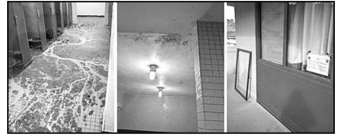
Junior-enlisted troops without dependents typically live in military-managed barracks. A Government Accountability Office report in September 2023 found some barracks pose serious health and safety risks. GAO investigators observed conditions such as sewage overflow, mold and mildew, and broken windows and locks. DoD photo courtesy Government Accountability Office
