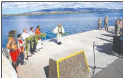
Kahu Kordell Kekoa performs a traditional Hawaiian blessing in August 2023 as the Navy begins construction on a new dry dock at Pearl Harbor Naval Shipyard and Intermediate Maintenance Facility. U.S. Navy photo Justice Vannatta
